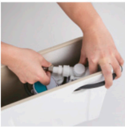
The water inlet pipe extends from the hole at the back of the water tank
